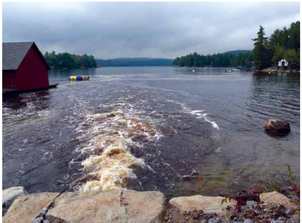
Figure 5. Stormwater flowing into Lake Sunapee, New Hampshire, through a road culvert. Photo: Midge Eliassen.
